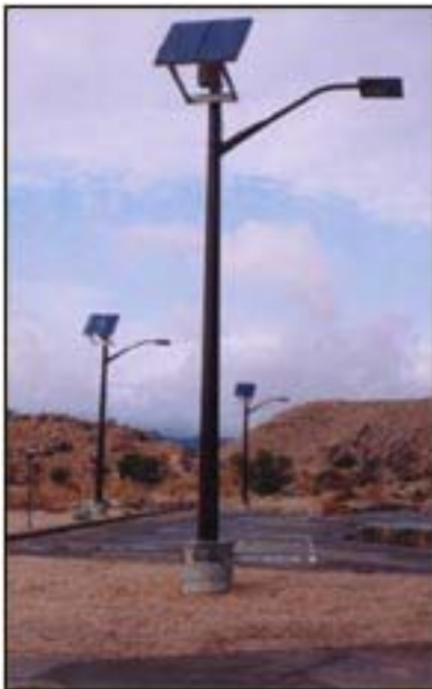
Figure 17. Solar parking lot lights.
