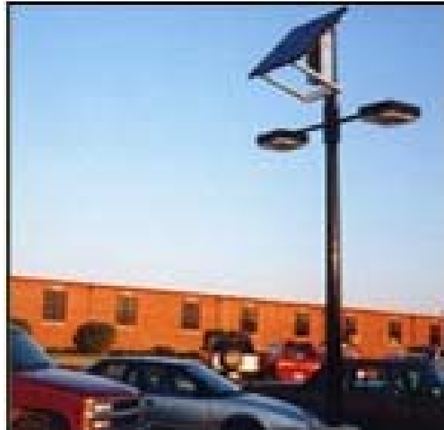
Figure 18. Solar parking lot light.
